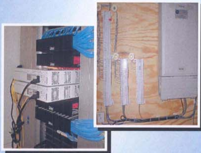
Photos Above Depict Installations by HNC
